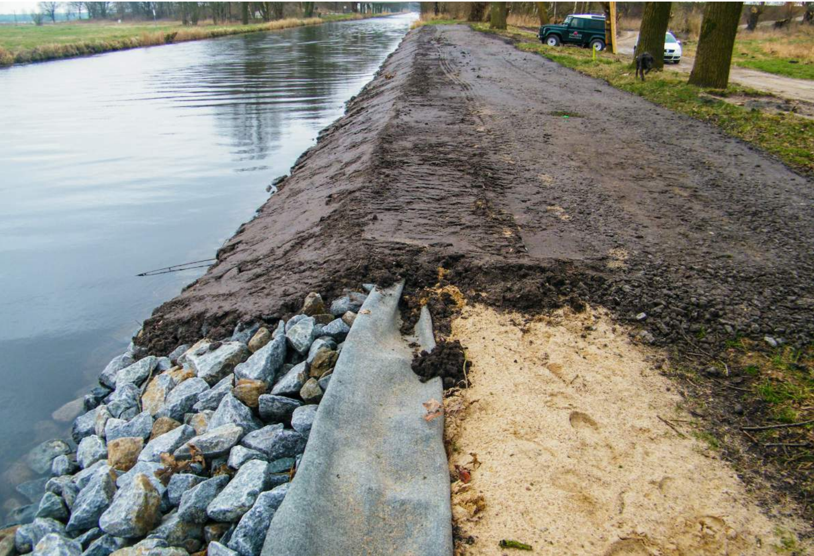
PHOTO Installation of armour stones and covering of the dam crest with humus sand or lean grassland and gravel.
